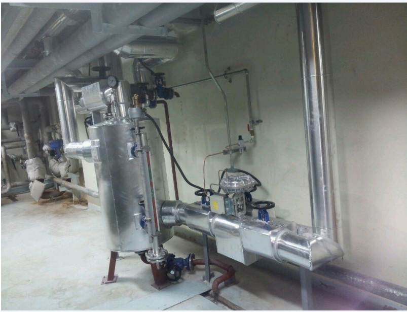
The installation: the new flash vessel and its piping.
